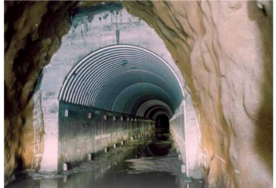
Fig. 18. The tunnel from Lake Päijänne was repaired for the first time in 1999. The reinforcement method used here is an exception and only used in cases of severe collapse. Some parts were bolted and shotcreted while most parts are still without any reinforcement. (Photo: Foto Mannelin Oy)
