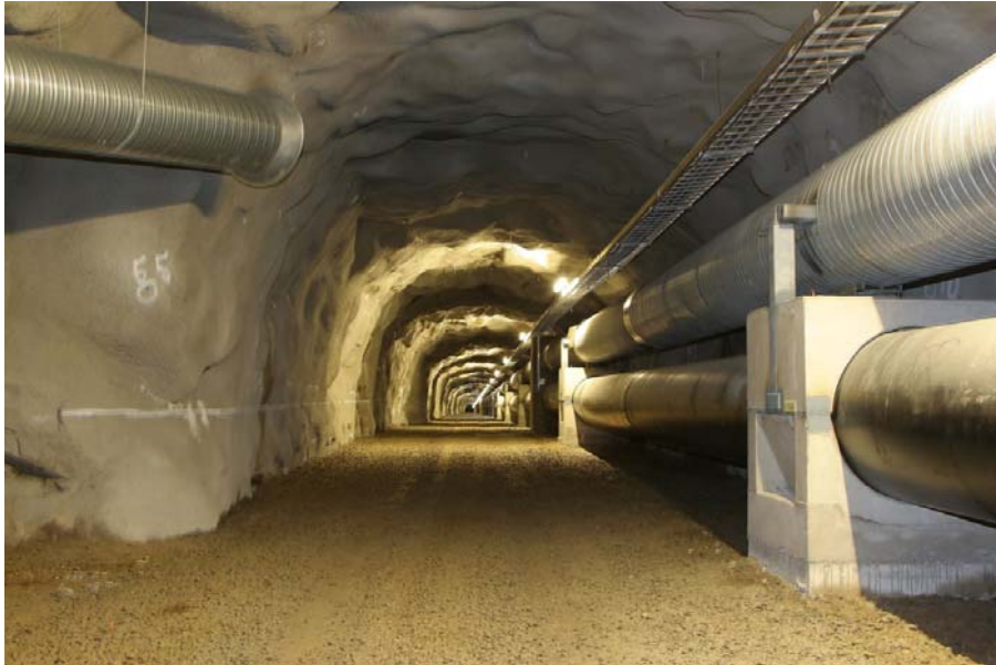
Fig. 10 Typical Utility Tunnel. (Photo: Jorma Vilkmán).
