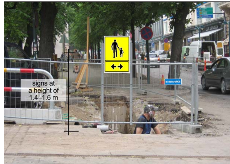
Figure 3. Worksite signs or their mounting posts/bases must not cause a risk of collision, falling or tripping.
